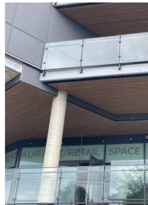
HORIZONTAL CEMENT BOARD SOFFIT SUPPLIER: WOODTONE (JAMES HARDIE) COLOUR: ASPEN RIDGE-RUSTIC SERIES
